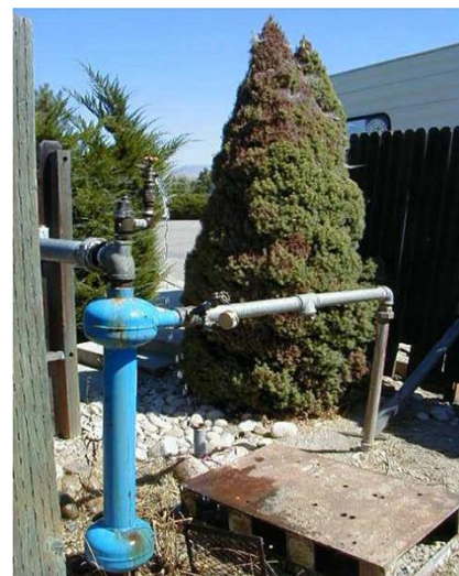
Figure: The wellhead on your property will typically include a pipe leading to your pressure tank.
